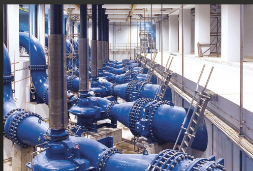
Pumps and compressors
